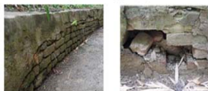
Broken brick masonry and plastering, mainly due to poor workmanship during construction and less maintenance
