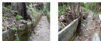
Damage to concrete channel by growing tree / roots
