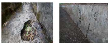
Broken floor slab mainly due to poor workmanship during construction
