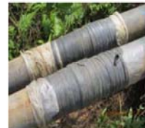
Rapping at leakage point (Temporary measure)
