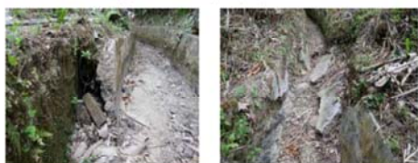
Collapsed canal section
