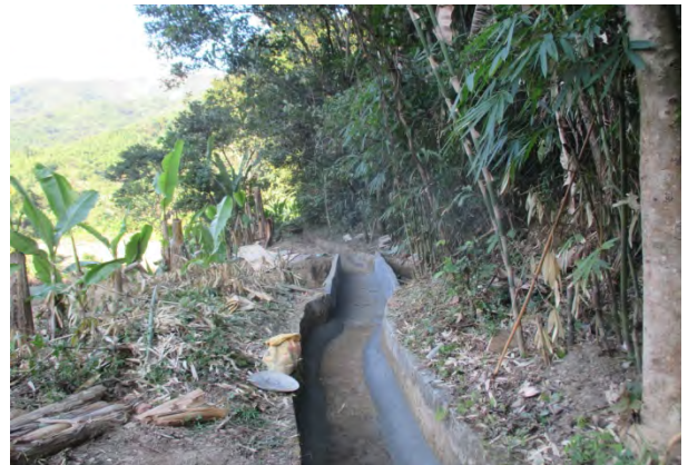
Construction of Aqueduct: Due to over flow from channel wall erosion occurred at the channel bed.
