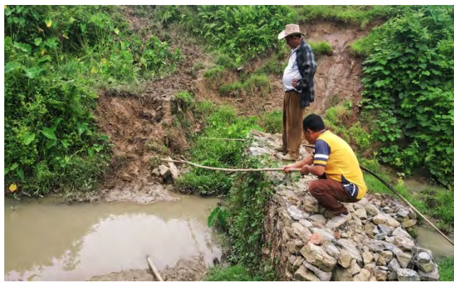
Checking the condition and effectiveness of check dam construction by the field officers from LRS&WCD
