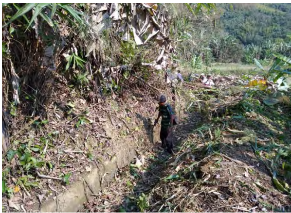
Community construction work for cleaning and desilting sand deposit from the channel
