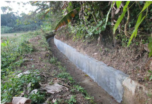
Channel walls repaired to prevent many leakage of water from the broken walls
