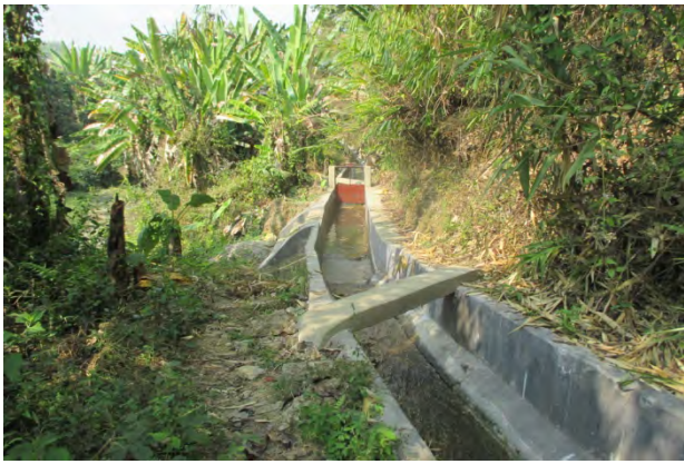
Maintenance of Main channel and construction of desiltation tank by contractor work
