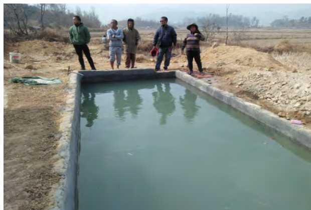
Water tank was constructed in WRC area to meet the farmers need for watering Rabi crop during winter season
