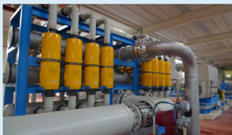
Photo 6—Pressure Exchange Skid
