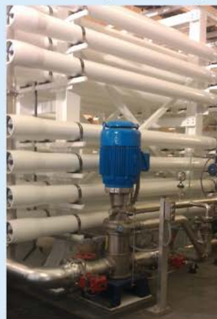
Photo 5—Motorized Turbocharger on RO Skid
