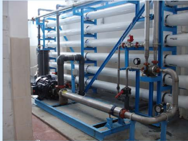
Photo 3—Small Turbocharger on RO Skid
