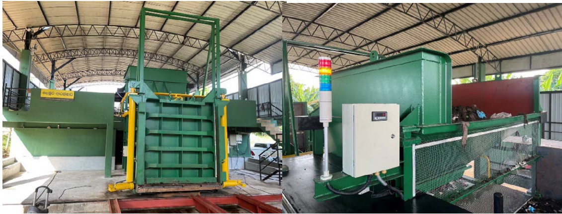
Figure 7 Waste container and hopper
