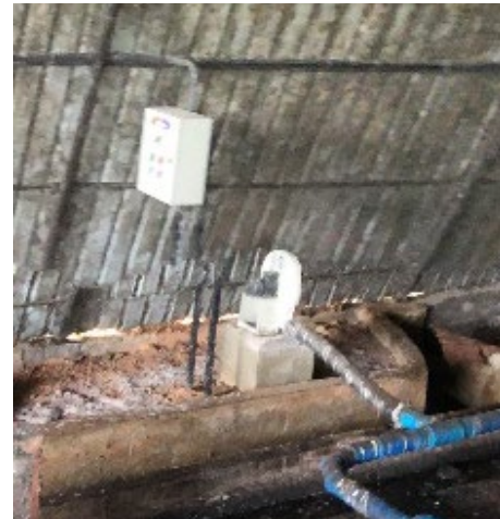
Figure 4 Blower and power supply
