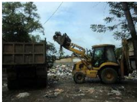
Gampaha MC Waste transfer is entrusted to a private company. Waste is transferred three times a day by 20 m 3 dump trucks.
