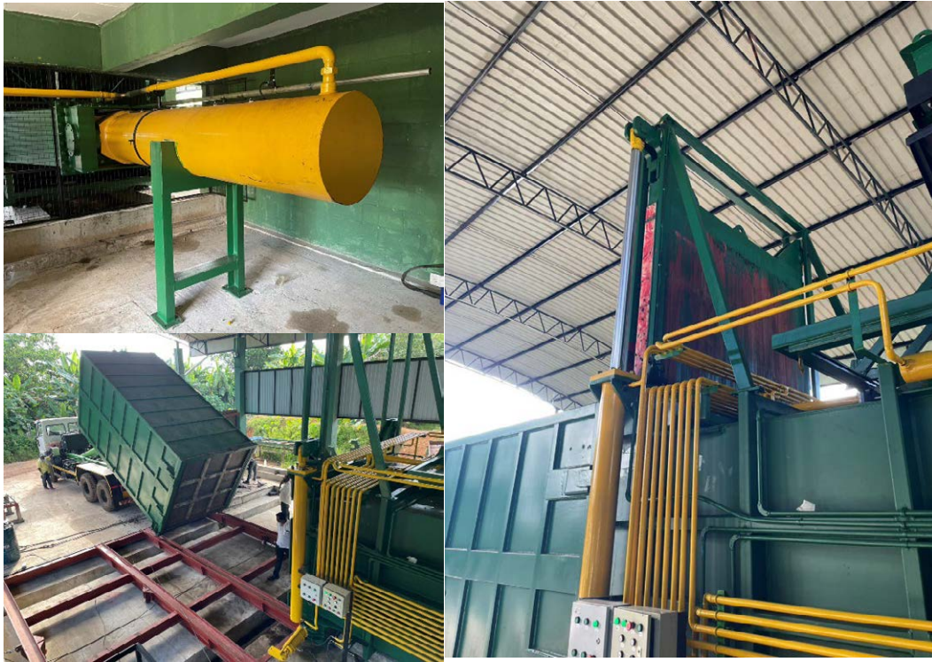
Figure 8 waste hydraulic compactor and container
