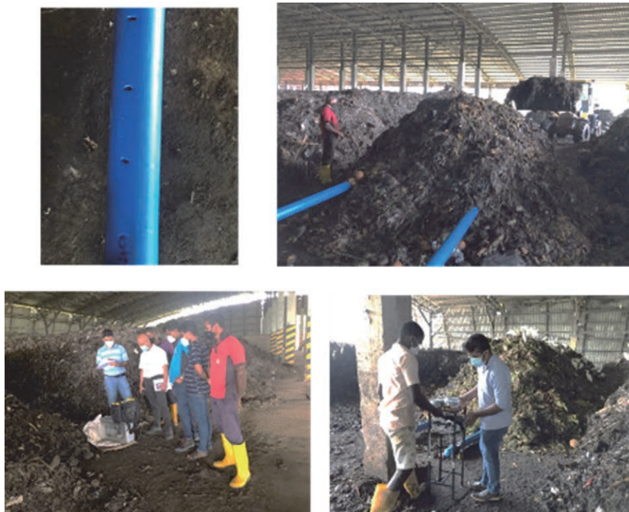
Figure 4-49 Aeration system and perforated pipes, performance measurement
