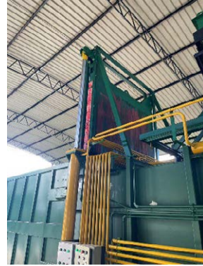
Compactor door lifting hydraulic cylinder
