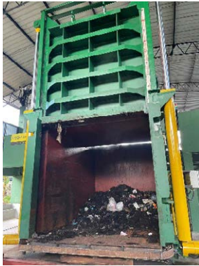
Solid waste container
