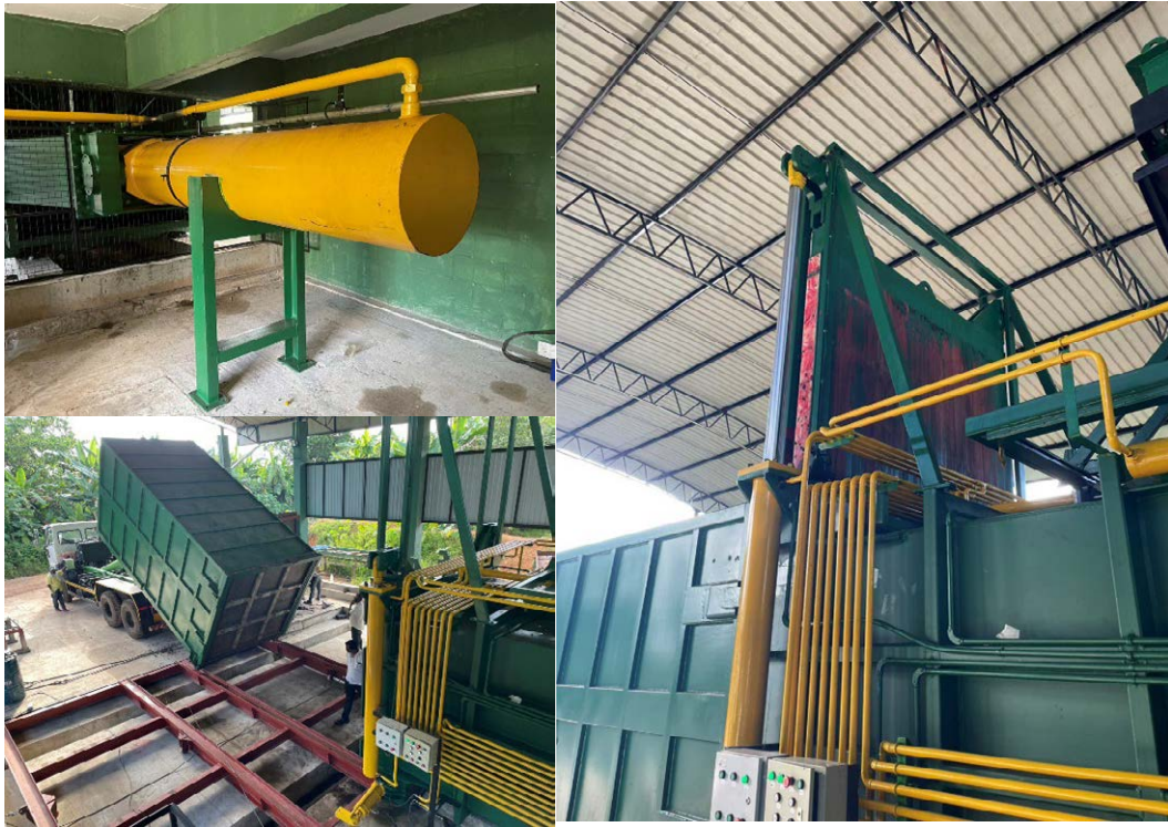
Figure 8 waste hydraulic compactor and container
