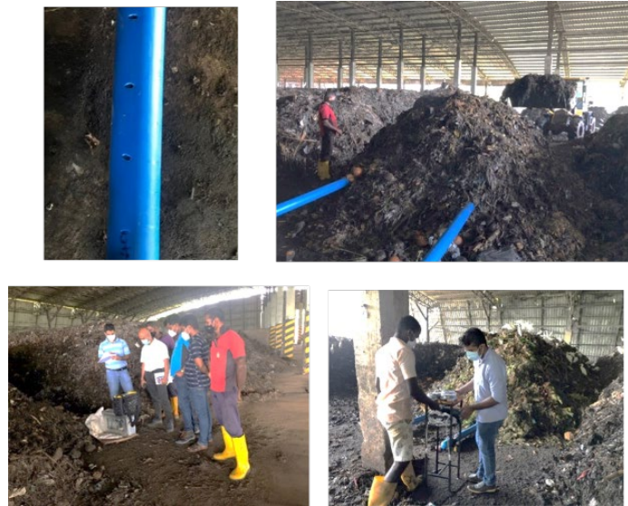
Figure 6 perforated pipe for air supply
