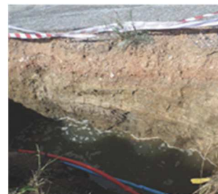
Photo: Existing fibre cable
