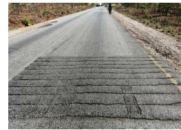
Photo: Rumble strip
