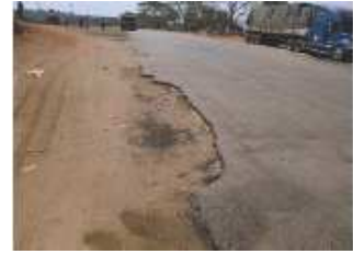
Photo: Status of erosion
