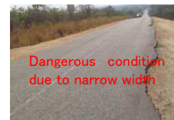
Photo: Road edge damage
