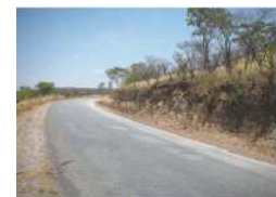
Photo: Insufficient sight distance spot
