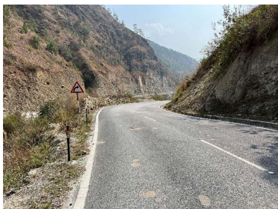
Road situation (Mongar side )
