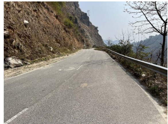
Road situation (Mongar Side)
