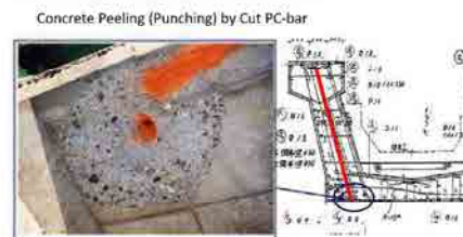
Concrete Peeling (Punching) by Cut PC-bar
