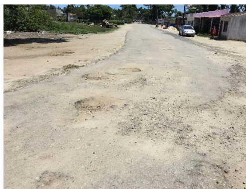
At Inhamizuwa and Chingussura. Many pavement surface areas were lost due to the deteriorated pavement.
