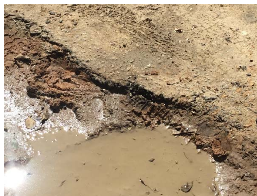
Pothole. The base and subbase were not found. The pavement surface might be constructed on the grand directly.
