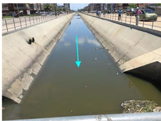
(3) No damage to the open channel
