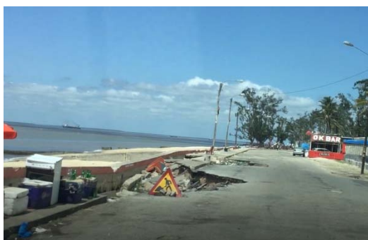
Damaged shoulder and sidewalk due to collapsed coastal protection
