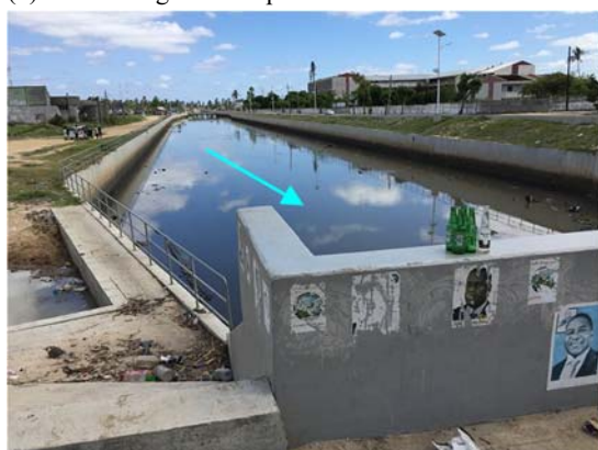
(5) No damage to the open channel around the upstream section of the watergate
