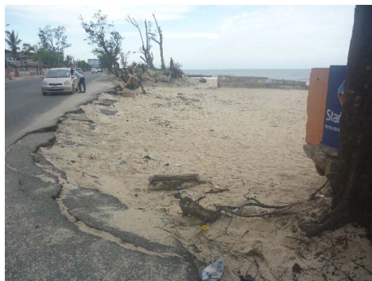
B) Damages of the seawall and coastal road
