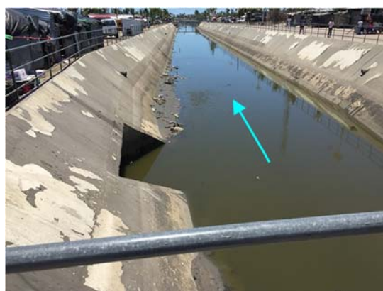
(4) No damage to the open channel
