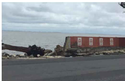
Lost road shoulder due to collapsed coastal protection
