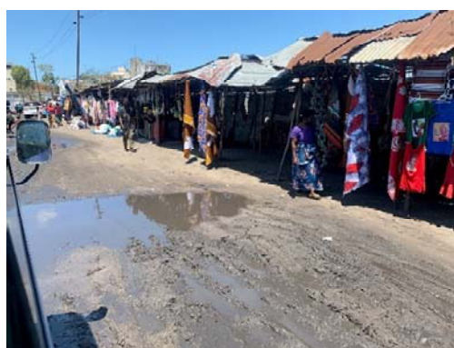
The road is barely wide enough for cars to pass each other. Water gathers in depressions and remains for several days, even after light rainfall.
