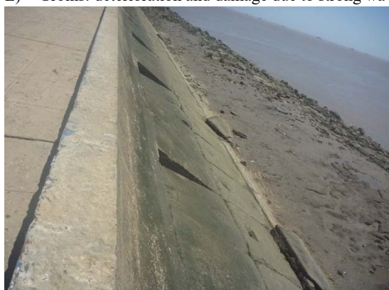
G) Hollowing-out in seawall
