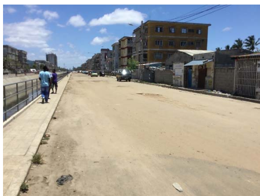
At Avenida 24. There were some potholes.
