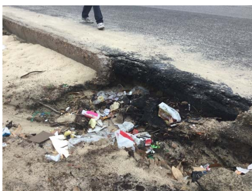
Damaged concrete block
