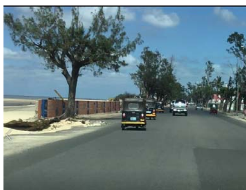
Loss of road shoulder due to collapsed coastal protection
