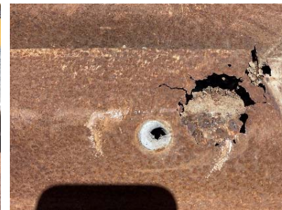
(f) Corrosion of existing roofing
