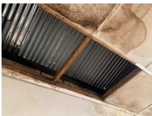
(a) Corroding Ceiling Sheets
