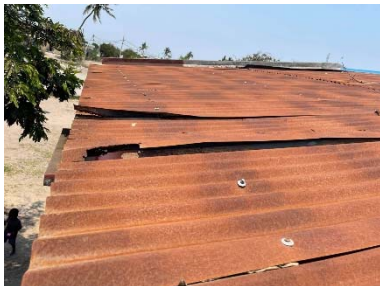
(a) Deformation/damage of existing roofing
