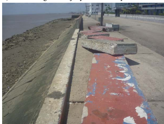
H) Damage of parapet near the port
