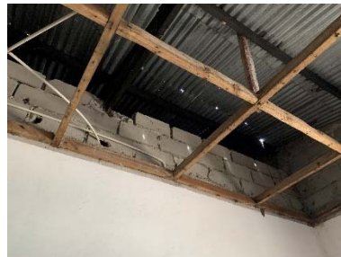
(b) Damage and gaps in existing roofing
