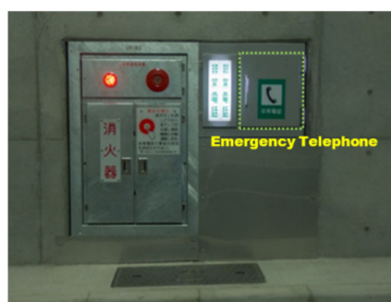
Emergency Phone on Wall
