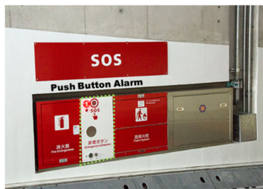
Push Button Alarm
