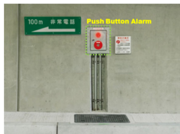
Push Button Alarm
