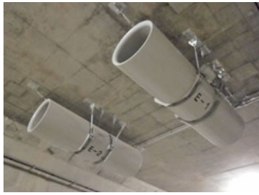
Smoke Removal System (Jet Fan)
