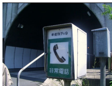
Emergency Phone at Entrance
