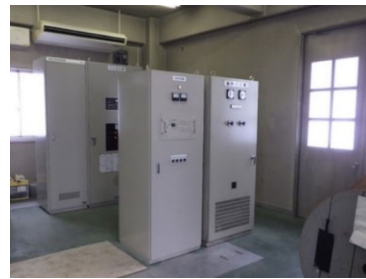
VMS Control Panel
