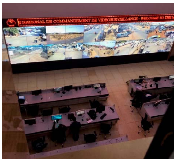
Control room in CCC
