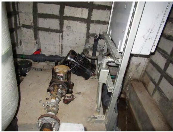
Water Supply Pressurized Water Pump The water supply pressurized water pump is failed and the motor section has been left disassembled. Currently, the system has been converted to a direct water supply system, instead of using a receiver tank and pressurized pump.
