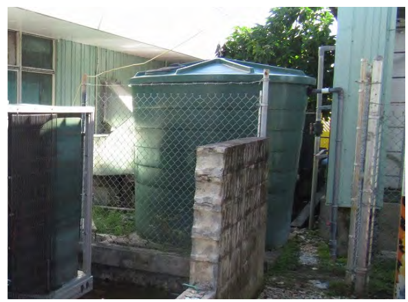
Seawater Receiver Tank The pump has failed, so the receiver tank is not in use, and the water is being supplied to the building via a direct connection to the water supply pipe, but the water is cut off due to a lack of water pressure.
