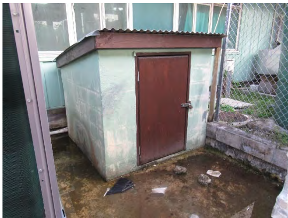
Seawater Pressurized Feed Pump The hospital reported that a seawater pressurized water supply pump installed by the hospital is located in this shed, but it has failed and is not in use.
