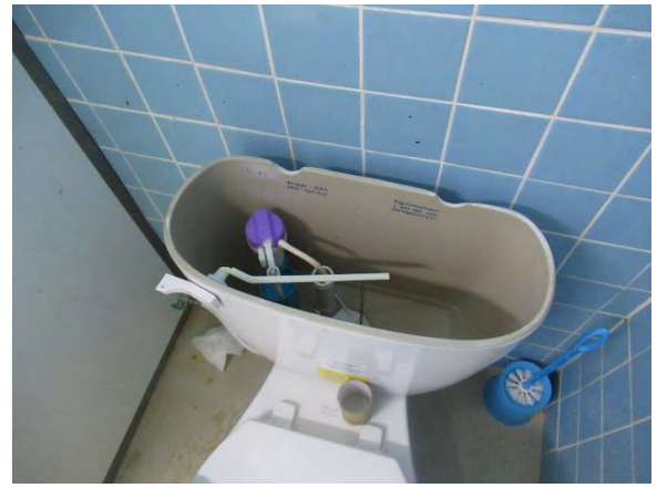
Building 1 In the lavatory on the 2nd floor (2) There is no water at all in the low tank of the closet bowl, and it can be assumed that the water has been cut off for some time.
