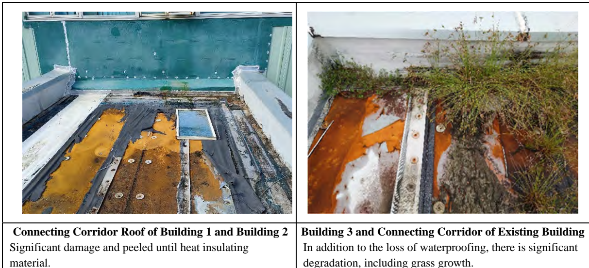
Figure 2-5: Corridors, Photographs concern with Roof Leaks
