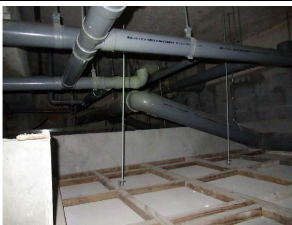
Building 1 In the ceiling under the lavatory on the 2nd floor (1)
