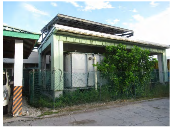
Water Supply Receiving Tank The water supply receiver tank has rust on the frame externally, but appears to have no problem with water storage performance. However the water supply pump has failed and is not in use.
