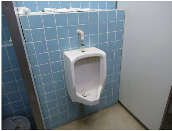
Building 1 In the lavatory on the 2nd floor (1) Men's lavatory. The washbasin provides water, but the urinal has the water supply connection removed and is unavailable.
