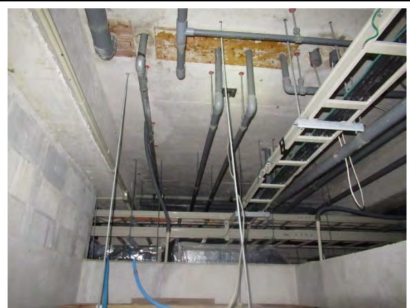
Building 1 In the ceiling under the lavatory on the 2nd floor (2)
