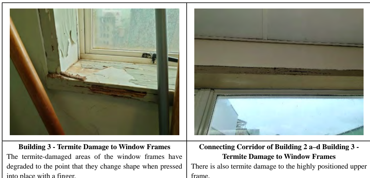
Figure 2-14: Photographs of Termite Damage
