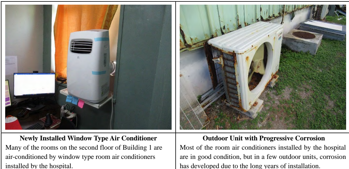
Figure 2-7: Photographs concern with Air Conditioning Equipment
