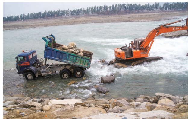
Photo 7.9 Repair Work of Riverbed Scouring due to Torrents at the Ends of Apron and Sand Flushing Ditch 1)
