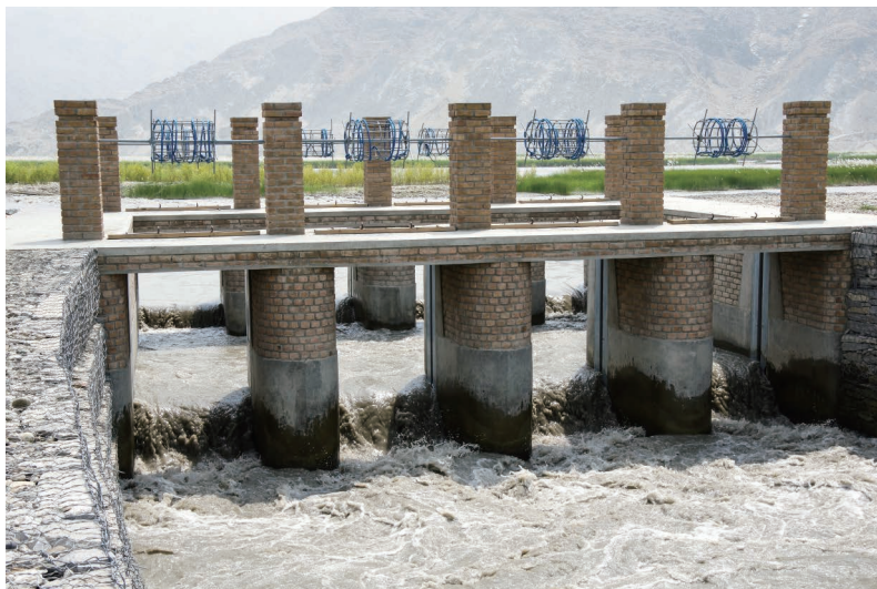
Photo 7.1 Double Flush Board Type of Intake Gate. Overflow Water Falls Stepwise. 1)
