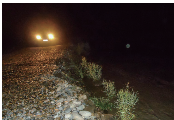
Immediately before the emergency work, a part of the top of the dike was flooded. The work was carried out desperately. July 17, 2015 7:30 pm
