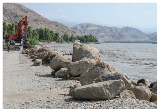
Prevention work of erosion by boulders was carried out throughout the night. Currently, the entire top of the dike is being raised. July 20, 2015
