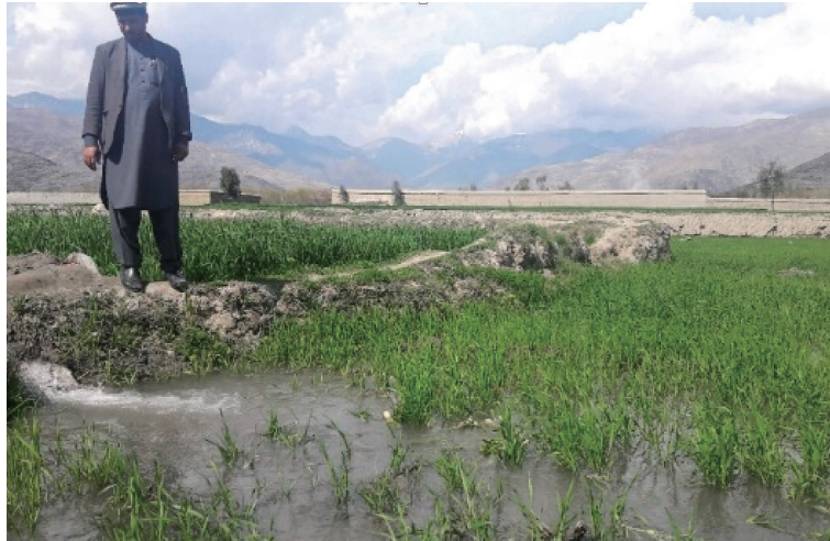
Photo 8.1 Damage Caused by Water Pressure at the Water Outlet 2)
