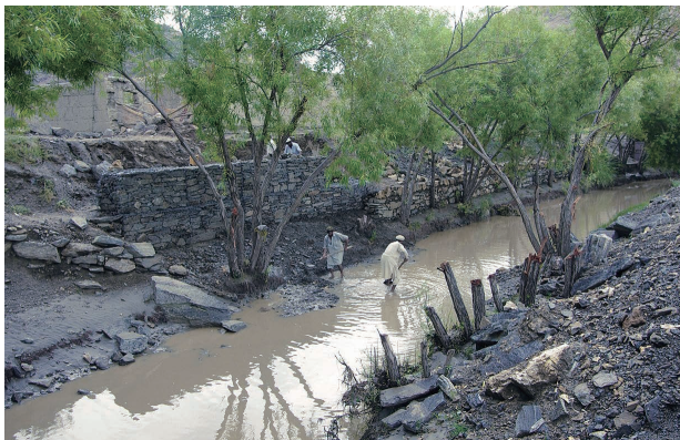
Photo 7.13 Destruction of Main Irrigation Canal Due to a Flash Flood and a Debris Flow 1)
