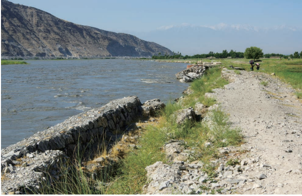
Photo 7.10 Riverbank Erosion Due to Flood Flow 1)
