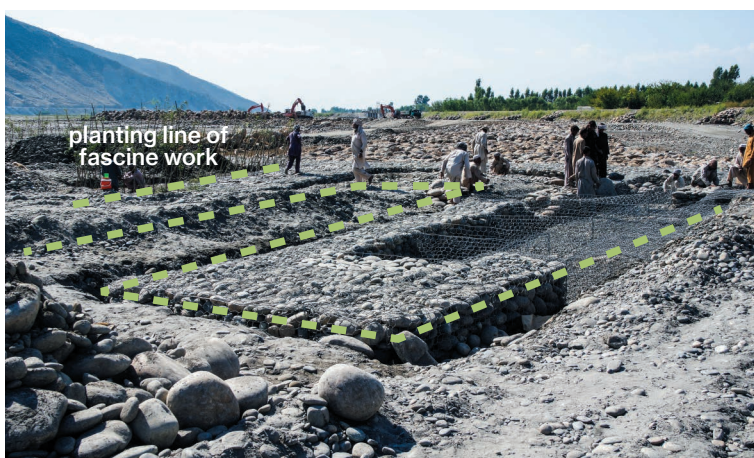
Photo 6.11 Gabion Works and Fascine Revetment (Wicker) Works for Sand Bar Protection (Miran) 1) : October 22, 2015
