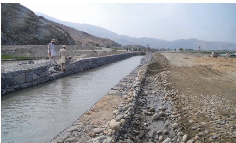
Photo 6.35 Piling up the Canal Revetment by Gabion Works (Marwarid II Main Irrigation Canal) 1) : July 18, 2018
