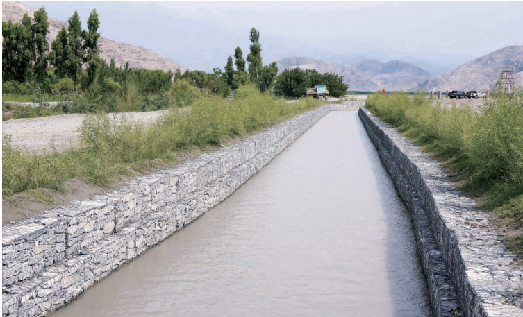
Photo 6.39 Wicker Works in Three to Four Months after Planting (Miran Main Irrigation Canal) 1) : September 21, 2015
