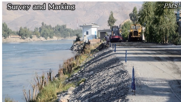
(1) Preparation works: determine the longitudinal location of the intake weir/gate. (Kama Weir I)
