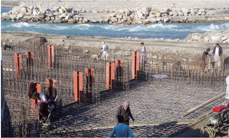
Photo 6.21 Reinforcement of the Bottom Slab and Gate Piers (Kama Weir I Sand Flushing Ditch) 1) : December 25, 2018
