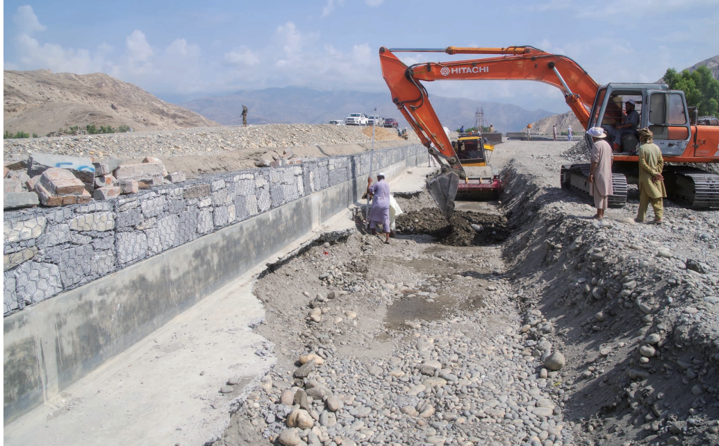
Photo: Collapse of Main Irrigation Canal Bed 1)
