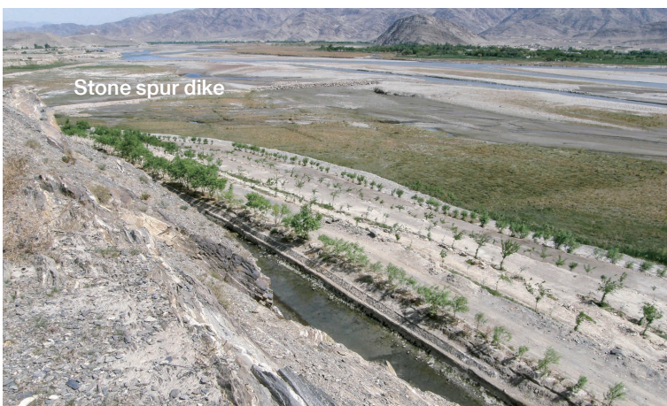
Photo 6.41 Irrigation Canal and Stone Spur Dike on the revetment (Marwarid Main Irrigation Canal, FG Section) 1) : March 24, 2008
