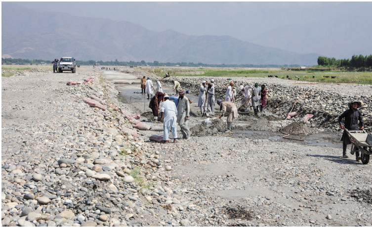
Photo 6.30 Under Construction of Soil Cement Lining and Other Canal Bed Works (Marwarid II Main Irrigation Canal) 1) : April 27, 2017
