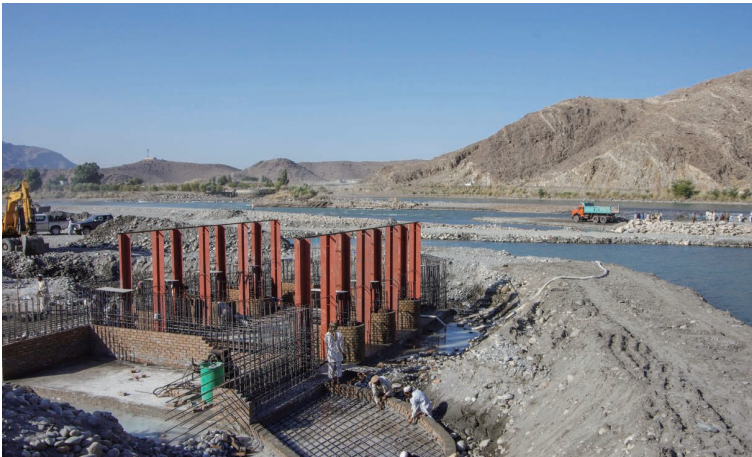
Photo 6.16 Gate Pier Reinforcement and Dry Construction Method by Temporary Cofferdike Applied to Intake Gate Construction (Kashkot Intake Gate) 1) :November 4, 2012
