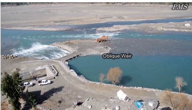
(9) Install a spillway when the water level is low during drought season. (Kama Weir II)
