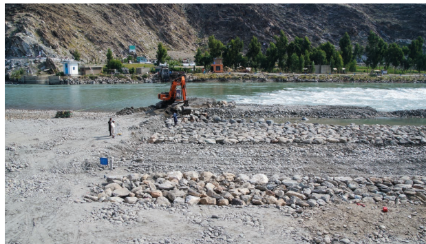
(8) Main civil works of intake weir: establish the intake weir body by piling up boulders from both side banks. (Kama Weir I)
