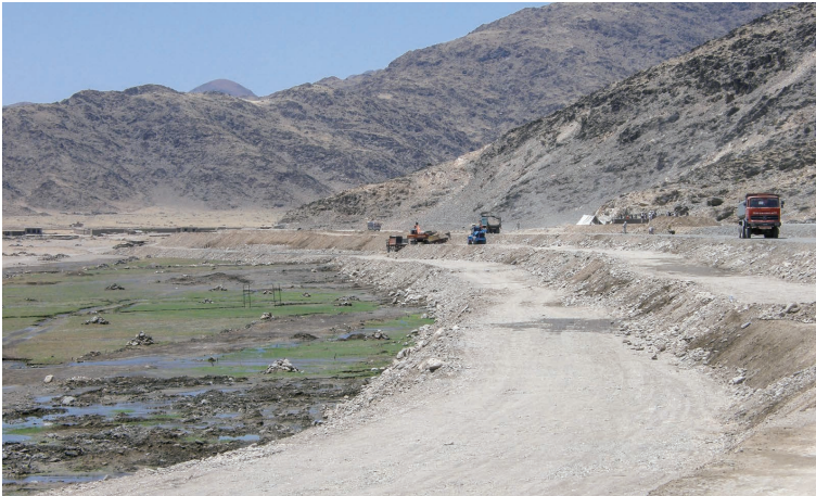
Photo 6.27 A Wetland is Formed below the Dike Embankment Slope by Seepage Water (Lower Left) (Marwarid Main Irrigation Canal Q2 Reservoir) 1) : June 28, 2009
