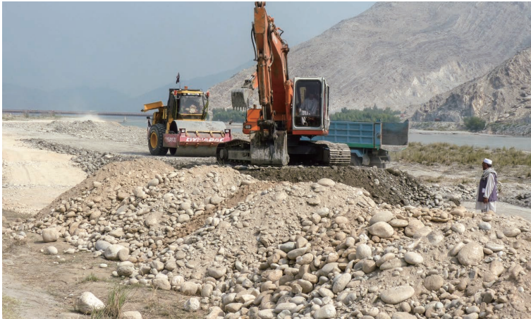
Photo 6.52 Unwinding and Rolling Compaction of the Embankment Materials (Behsud Bank Protection) 1) : October 13, 2010
