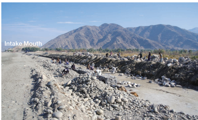
Photo 6.32 Creating and Laying Gabions (Lower Layer) (Marwarid II Main Irrigation Canal) 1) : December 18, 2016
