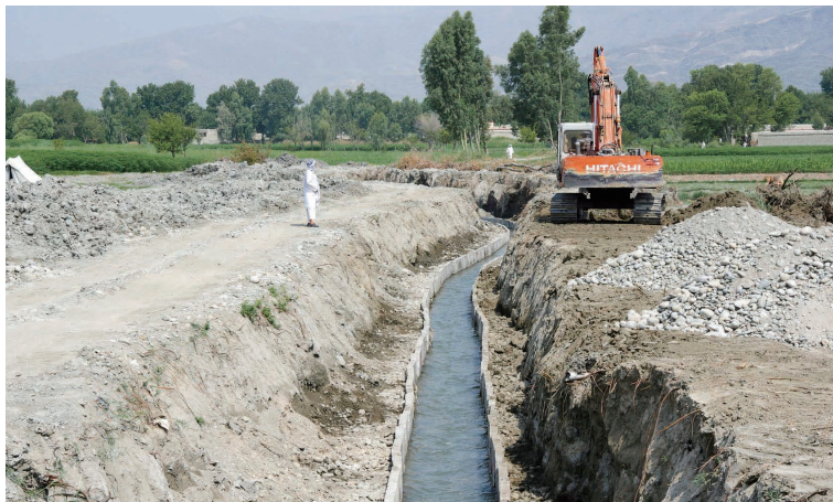
Photo 6.50 Installation of a U-shaped Canal in the Drainage Canal (Gamberi Main Drainage Canal) 1) : July 23, 2016
