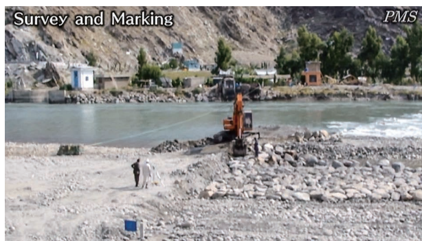
(3) Opposite bank reinforcement/revetment works: the intake weir wing on the opposite bank (attachment part to sandbar) is reinforced in advance. (Kama Weir I)
