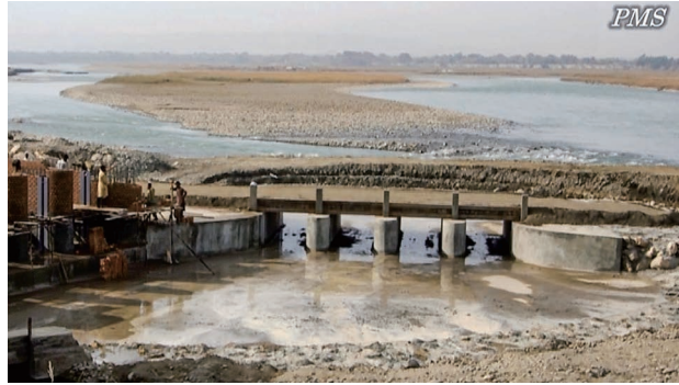
(6) Install temporary bridge on sand flushing ditch: for traffic of heavy machines used to construct the main body of intake weir. (Marwarid Weir II)
