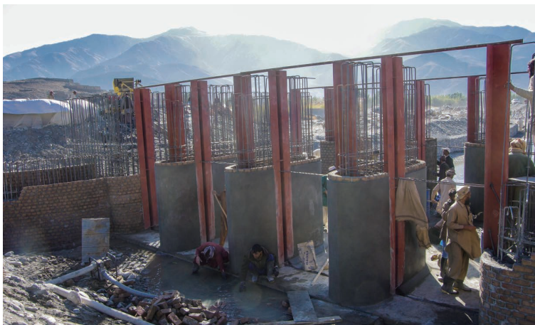
Photo 6.17 Structural Reinforcement of Gate Piers and Installation of Gate Ditch (Kashkot Intake Gate) 1) :November 15, 2012
