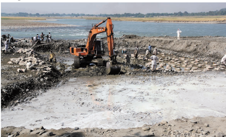
Photo 6.20 Construction of Spread Foundation 0.5 m or more Thickness (Marwarid II Sand Flushing Ditch) 1)
