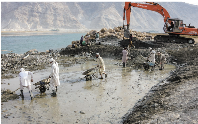
Photo 6.14 Construction of Spread Foundation 0.5m or more Thickness (Miran Intake Gate) 1) :November 24, 2014
