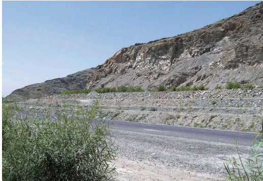
One and a half years after construction, wickers along the main irrigation canal (upper step) grow to 1.0 to 1.5 m in height. Mulberry trees on the second and third steps have just been transplanted with young trees. As of April 28, 2007.
