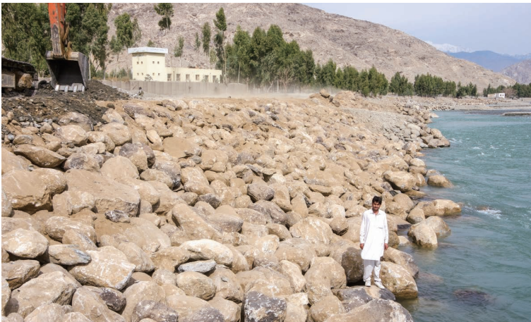
Photo 6.56 Inputting Stone Materials to Construct the Stone Spur Dike (Hundreds of Meters from the Miran Revetment Starting Point) 1) : February 12, 2015
