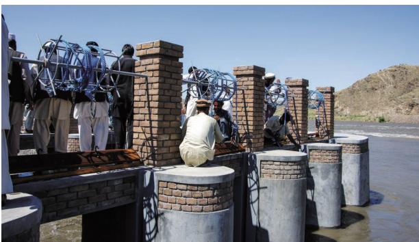
(11) Checking the performance of equipment works: check the performance of the double flush boards and lift-up equipment of intake gate and sand flushing ditch. (Kashkot Weir)
