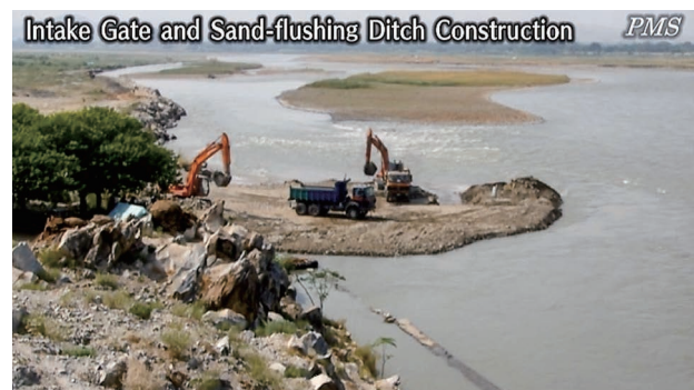
(4) Temporary works: construct a round temporary coffer dike surrounding the proposed intake weir, sand flushing ditch and sedimentation pool. (Marwarid Weir II)
