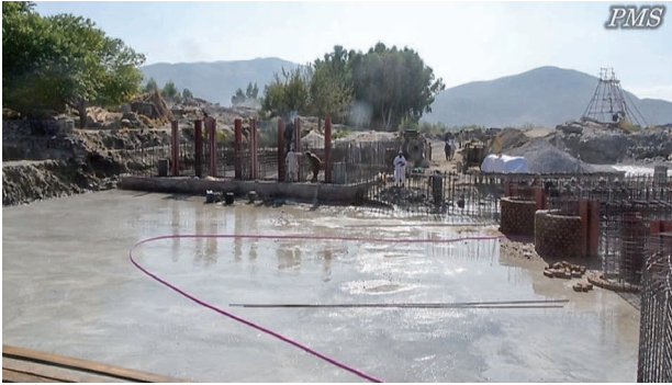
(5) Construction of intake gate, sand flushing ditch and sedimentation pool: carry out foundation works, main civil works, equipment works, revetment works and apron works. (Marwarid Weir II)
