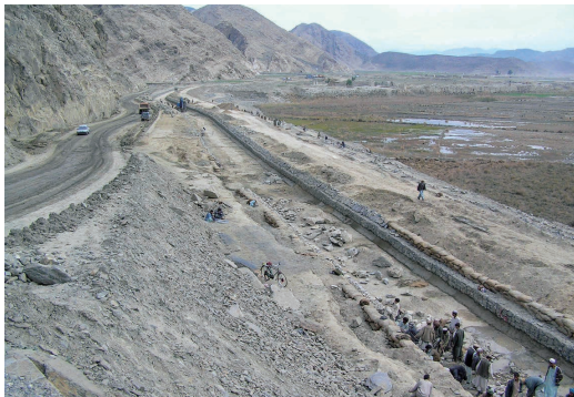
The canal on the embankment is under construction. Bedrock and wetlands are shown on the left and right sides, respectively. As of February 27, 2005.
