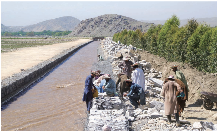
Photo 6.34 Creating and Laying Gabions (Upper Layer) (Marwarid II Main Irrigation Canal) 1) : April 8, 2019
