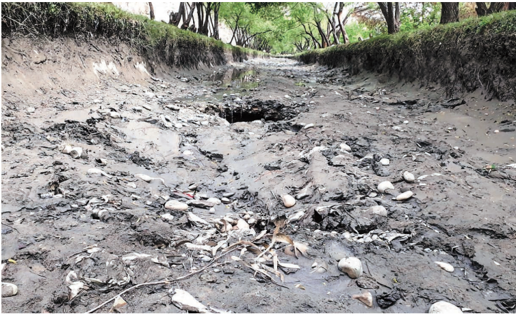
Photo 6.36 Occurrence of Piping on the Main Irrigation Canal Bed (Marwarid Main Irrigation Canal, FG Section) 1) : April 6, 2020
