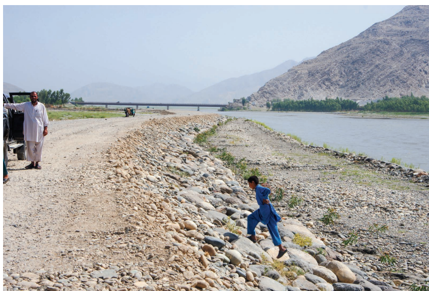
Photo 5.1 Stone Pitching on a Continuous Dike, Small Berm, and the Upper Slope of the Small Berm 2)
