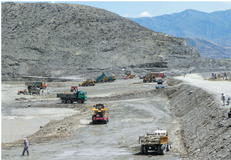
Photo 6.26 Heavy Machines, Dump Trucks and Workers in the Dike Embankment (Marwarid Main Irrigation Canal Q2 Reservoir) 1)
