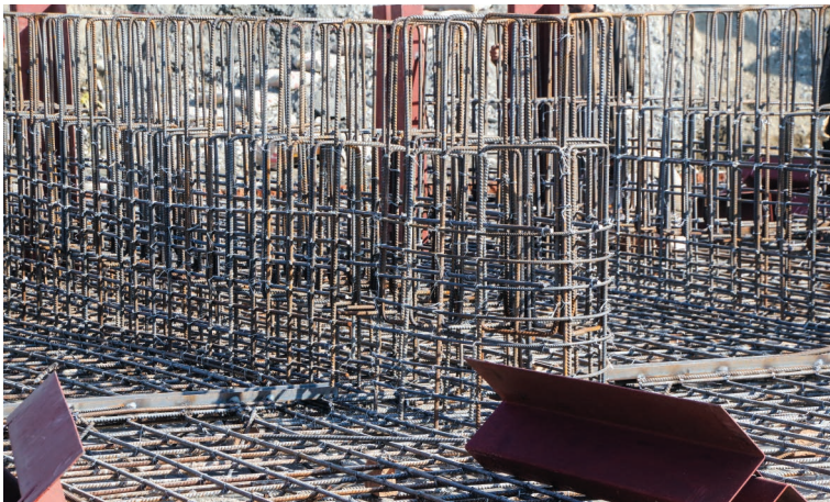
Photo 6.22 Reinforcement of Bottom Slab and Gate Piers in Detail (Kama Weir I Sand Flushing Ditch) 1) : December 24, 2018
