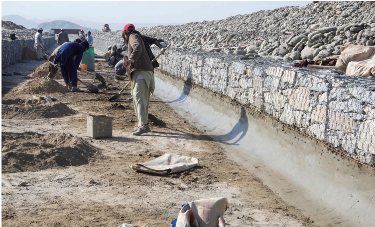
Photo 6.33 Filling Soil Cement in the Canal Bed Corner of Main Irrigation Canal (Marwarid II Main Irrigation Canal) 1) : December 24, 2016
