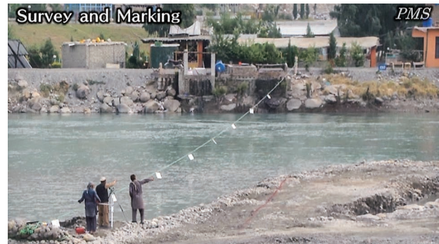
(2) Preparation works: determine the horizontal location of the intake weir/gate. (Kama Weir I)
