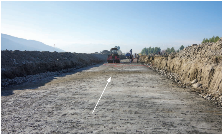
Photo 6.31 Soil Cement Lining Works on the Canal Bed (Miran Main Irrigation Canal) 1) : December 11, 2014
