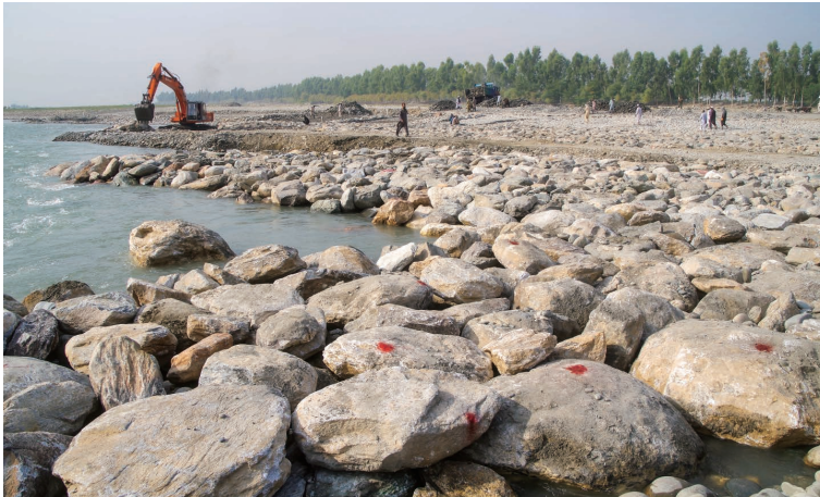
Photo 6.6 Stones with Height Mark for Piling up Boulders (Kama Weir I) 1) : October 29, 2018
