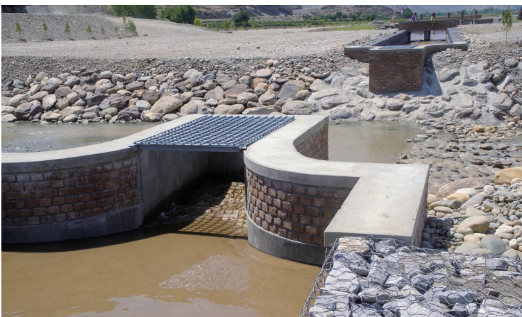
Photo 6.45 Safety Measures for the Siphon (Marwarid II Canal) 1) : June 30, 2018
