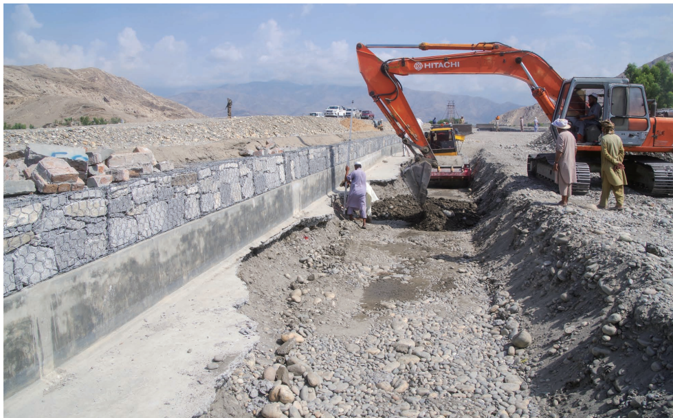
Photo 4.15 Collapse of Canal Bed due to Improper Foundation Condition 1)
