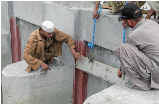
Photo 5cm-thickness iron plate is put in place and a hook is welded. A hook at the end of the rope is hooked and the board is lifted by a hoisting device. 1)
