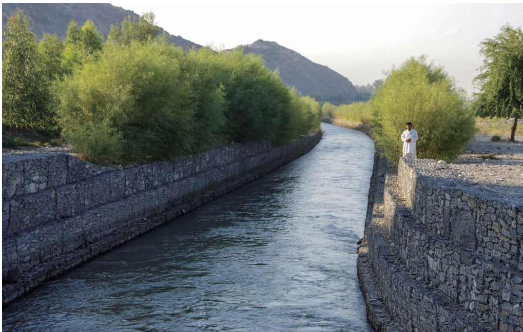
Photo 4.8 Example Gabion Works and Wicker Works in the Main Irrigation Canal 1)
