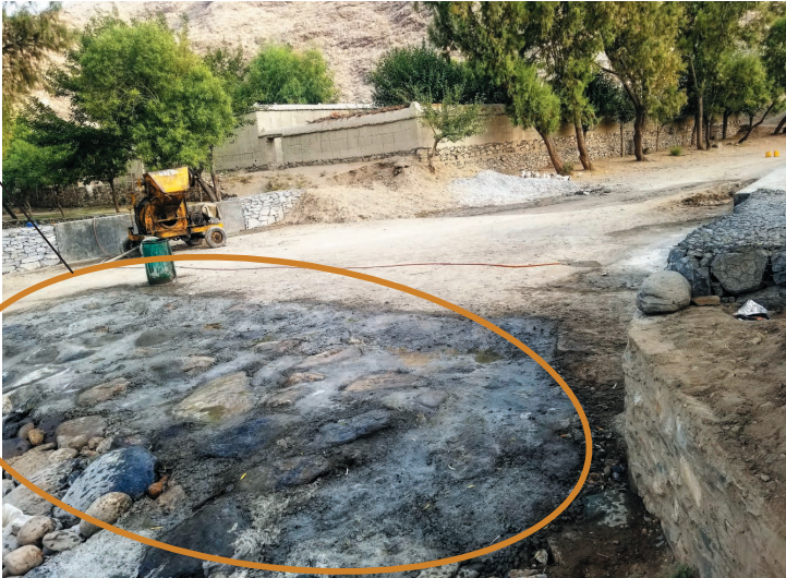
Photo 4.20 Connection Point of the Slab of the Flood Crossing Bridge to the Ground 1)
