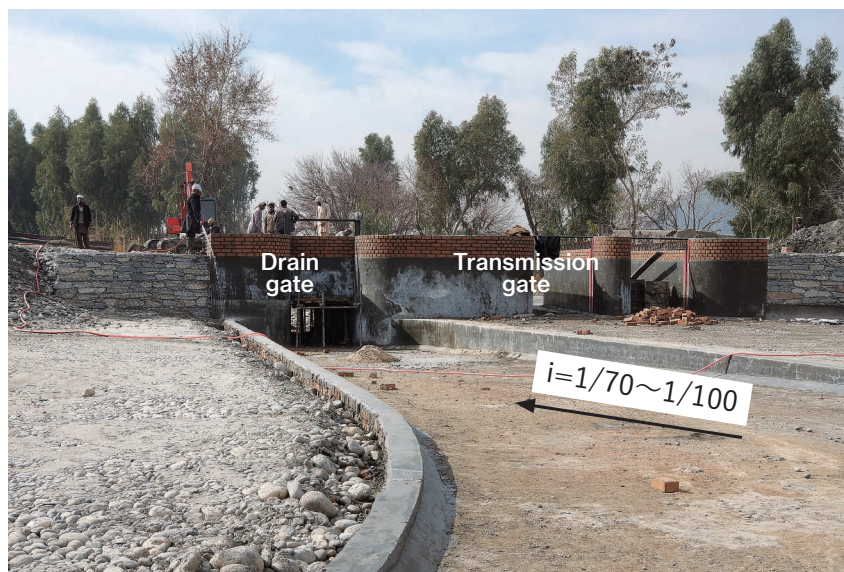
Photo 4.17 Concrete Sand Drain Canal at the Bottom of the Sand Basin and Drain Gate 3)
