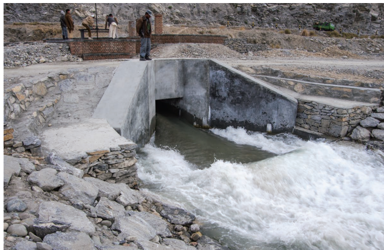
Photo 4.18 Drain Gate Outlet of the Sand Basin and Drain Gate Outflow from the Sand Basin 1)
