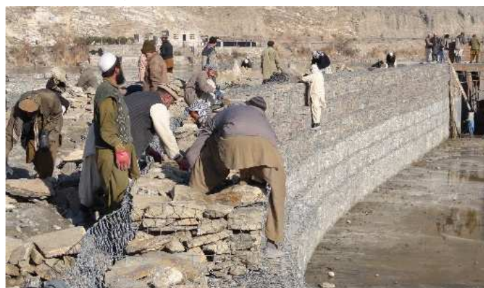
Gabion, which is one of the basic civil engineering techniques of the PMS irrigation project, is installed on the side of the canal.
