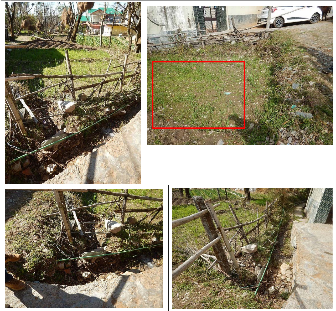
Current state of intake and open-channel and Place for underground water tank
