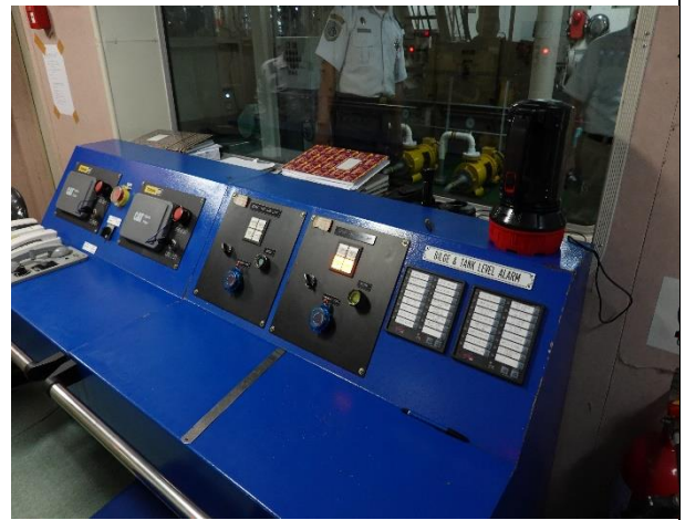
Photo 87 Tarakan Visit - KN Maratua Engine Room (2)
