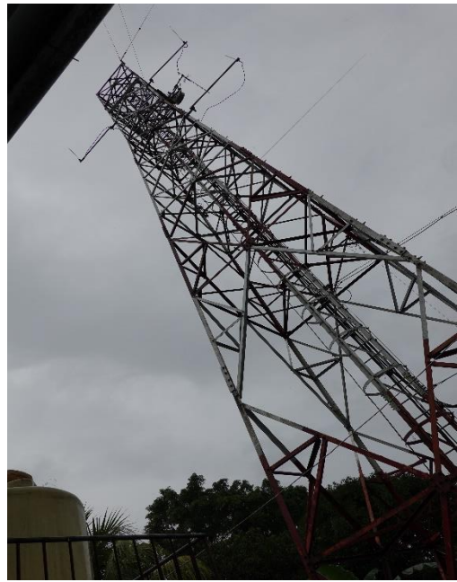
Photo 37 Ambon Visit - Radio Tower
