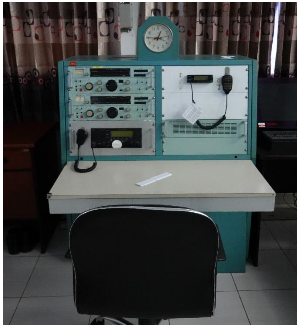
Photo 36 Ambon Visit - Inside Ambon Coastal Radio Station
