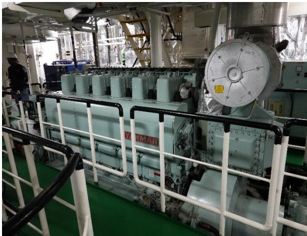
Photo 52 Ambon Visit - KN Bacan Main Engine (1)
