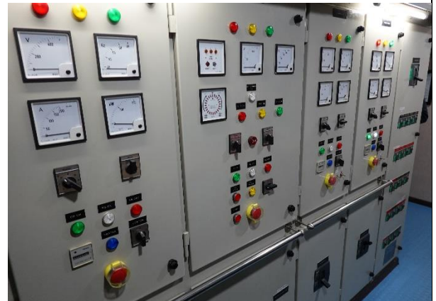
Photo 47 Ambon Visit - KN Bacan Engine Room
