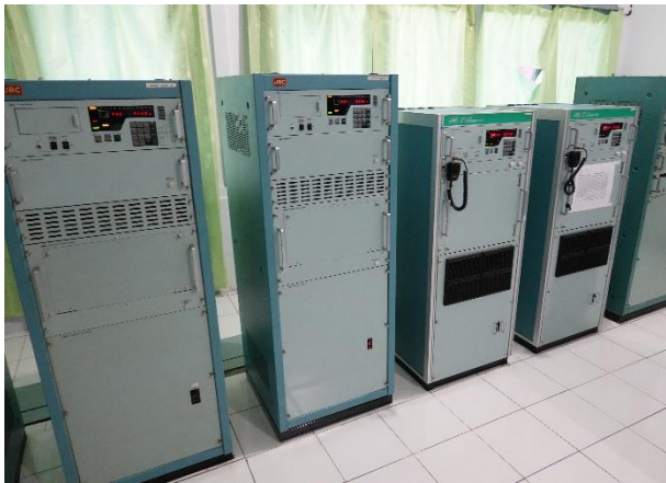
Photo 38 Ambon Visit - Inside Ambon Coastal Radio Station
