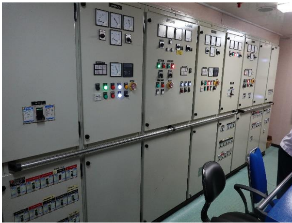
Photo 86 Tarakan Visit - KN Maratua Engine Room (1)
