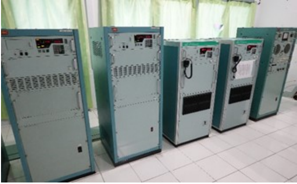
MF / HF transmitter
