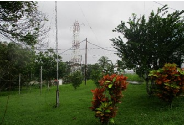
MF / HF antenna tower
