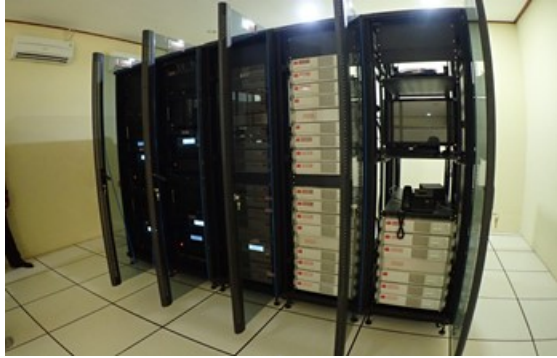
HF Transmitter Units
