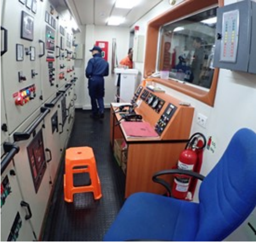
Engine console Room
