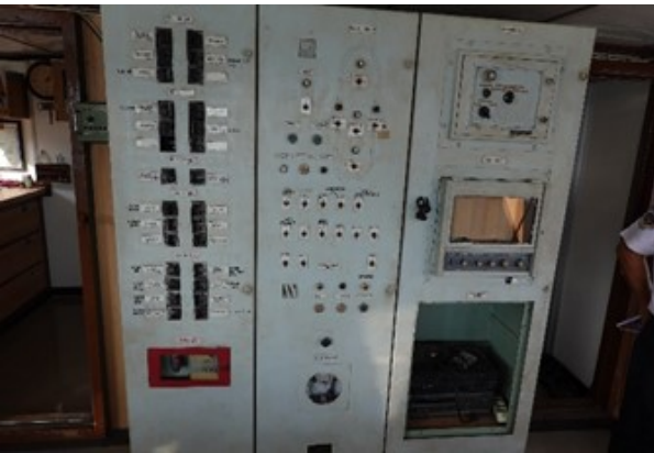
Operation power board
