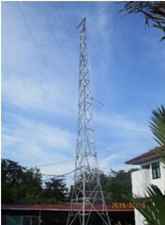
Antenna and tower
