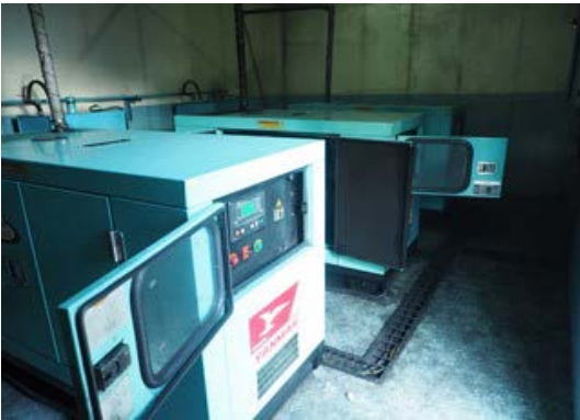
in-house power generator
