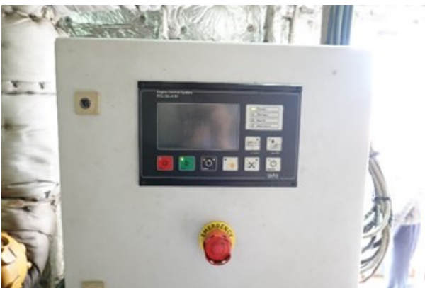
Spare engine control panel
