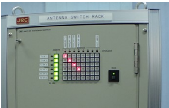
Antenna Switch rack
