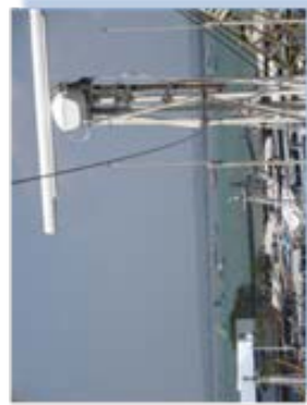
6 Feet Radar Antenna
