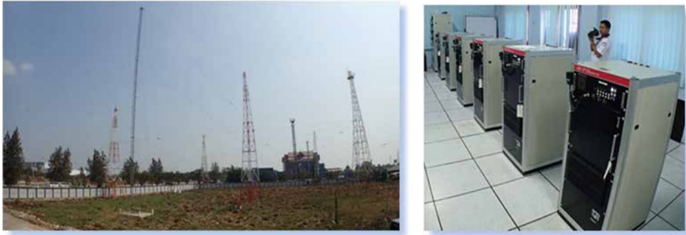
Picture 4.1.4 -2 : HF, MF Antenna Tower, Transmitter and Control Unit
