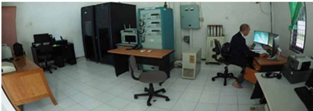
Picture 4.1.8 -7 : CRS Operation Room
