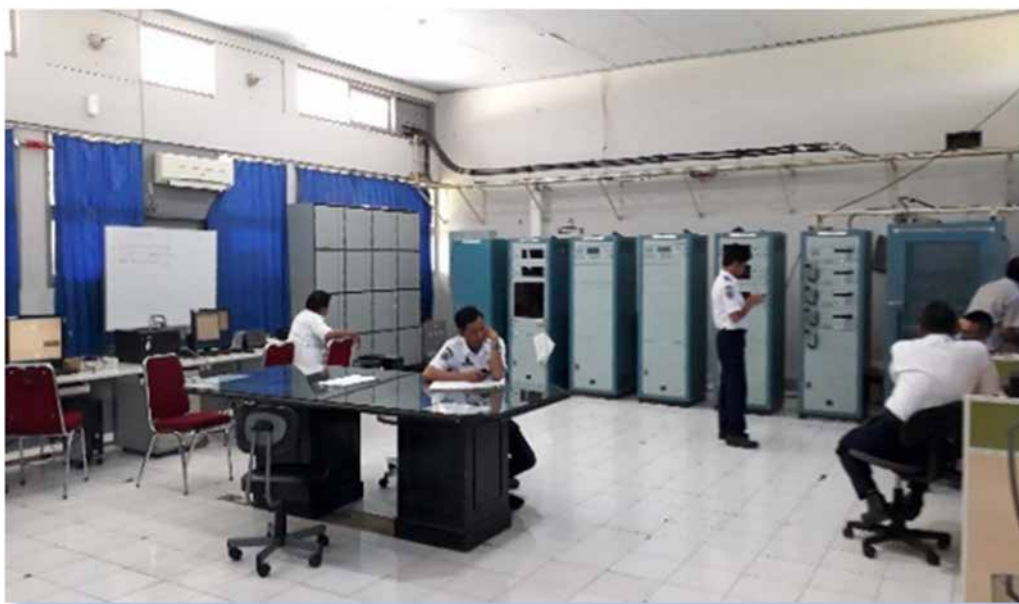
Picture 4.1.7 -3 : GMDSS Operation Room and Equipment
