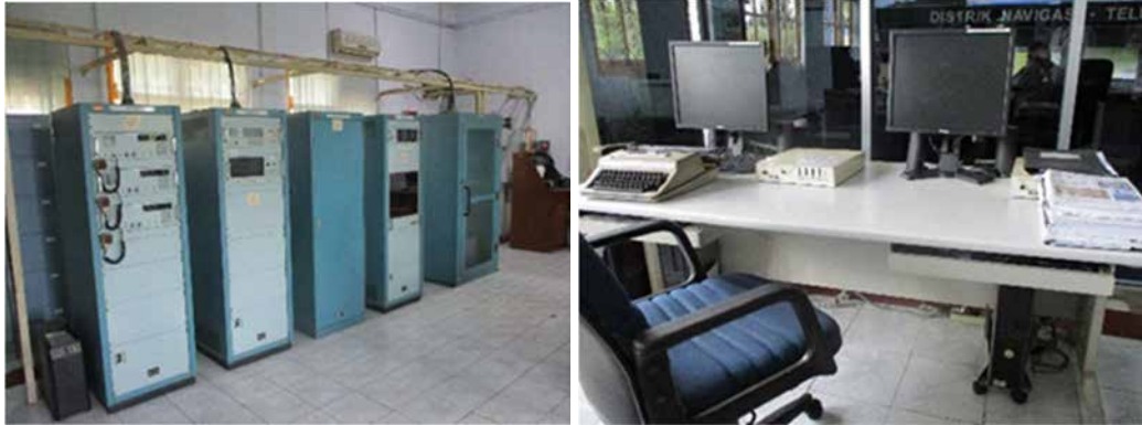
Picture 4.1.13 -5 : MF/HF, VHF TX/RX, GMDSS Console
