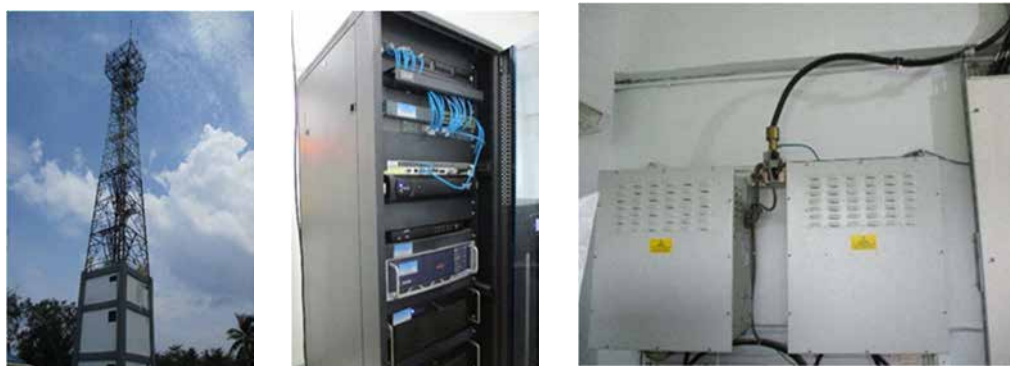
Picture 4.1.10 -4 : Tg. Intan unmanned sensor station
