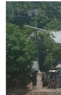
Flood Light Station *
