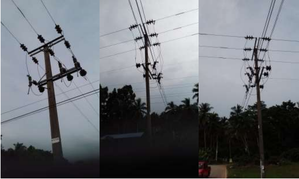
Isolator @46AVI-011 for TSS 6
