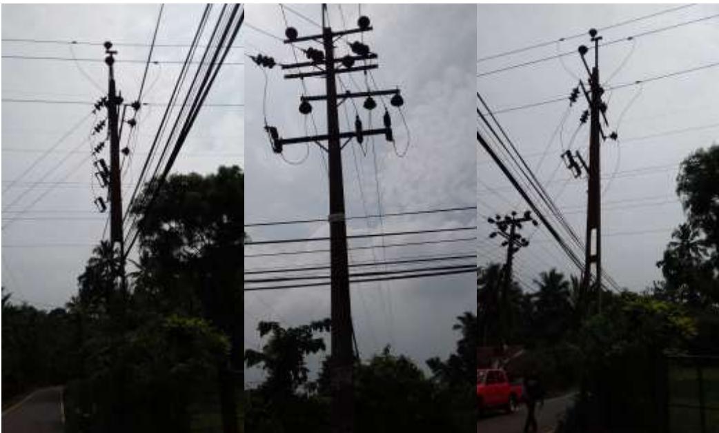
Isolator @46AVI-004 for TSS 1
