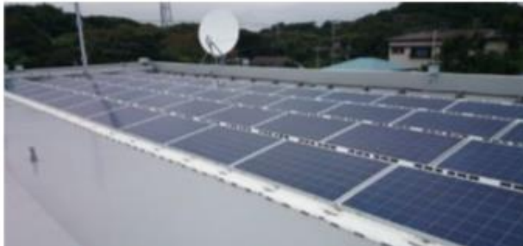
④ Small PV equipment + Storage battery equipment
