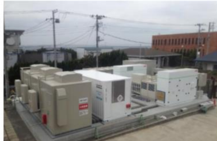
③ Storage battery equipment
