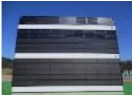
Example of PV installation on the wall of a building (NEDO)
