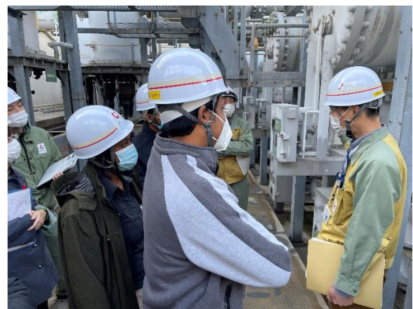
Visiting Nunoike Substation
