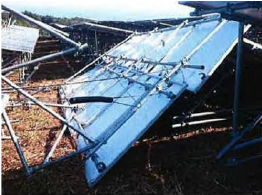
Collapsed solar panels
