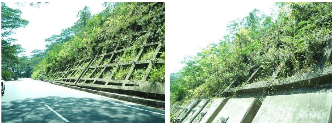
Figure 5-2 Concrete Crib Works Using Both Soil Nailing and Anchor Works by LDPP
