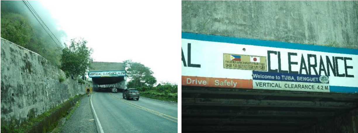
Figure 5-5 Rock Shed on Rosario-Pugo-Baguio Road
