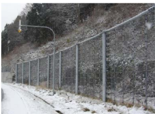
(a) Support Reinforced Fence
