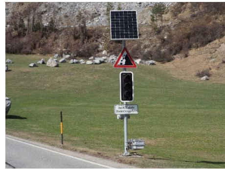
Signal connected to Doppler radar
