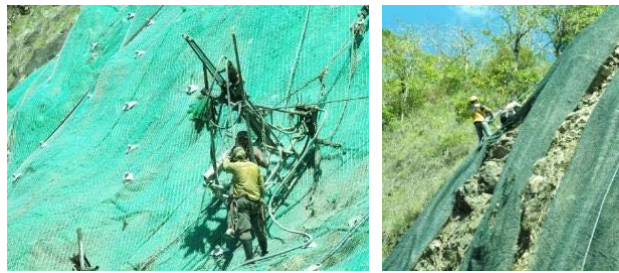
Figure 5-11 Drilling/Inserting Soil Nailing (left) and Removing Boulders before Placing Wire Mesh (right) in Philippines
