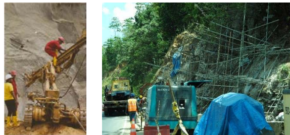
Figure 5-13 Drilling Work with Self-Propelled Boring Machine (left) and Drilling/Insertion of Soil Nailing with Single Pipe Scaffold (right) in Sri Lanka
