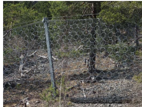
Rock fall fence (Switzerland)
