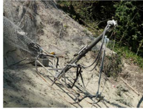
Very simple rotary percussion boring machine, fixed by wires on the slope.
