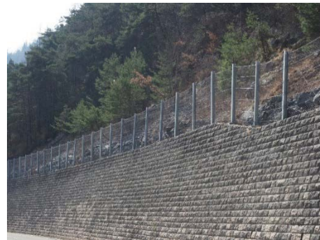
Rock fall fence with retaining wall (France)
