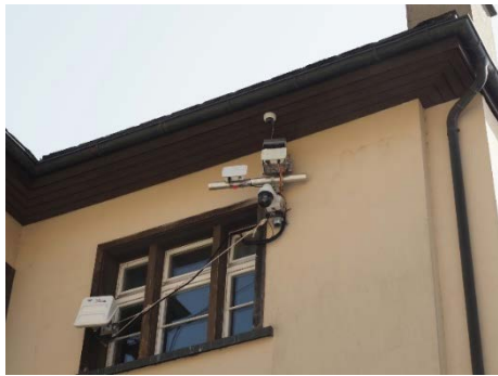
Doppler radar to detect fallen rocks
