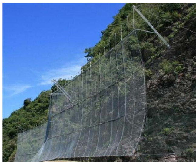
(b) High Energy Absorbing Rock Fall Net
