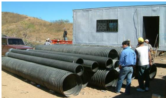
Photo 7-16 Leachate Collection Pipes
