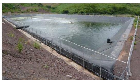
Photo 7-19 The Use of Aerators in the Leachate Pond
