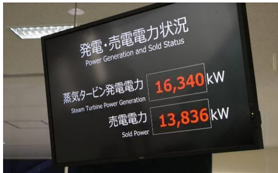
Photo 4-42 Monitor of Suginami Incineration Plant Showing Amounts of Power Generation and Sold Power
