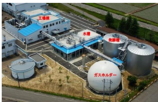
Photo 4-46 Methane Gasification Facility in Nagaoka City, Niigata Prefecture
