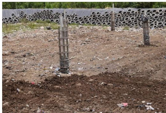
Photo 4-73 Gas Venting Pipes
