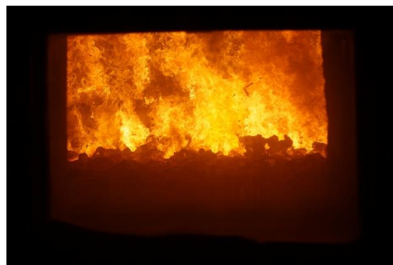
Photo 4-39 (9) Waste Incineration inside Stoker Furnace
