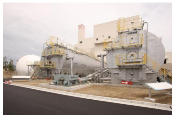
Photo 4-47 Methane Gasification Facility in Hofu City, Yamaguchi Prefecture
