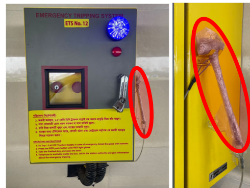
Source: JICA Expert Team Emergency Button
