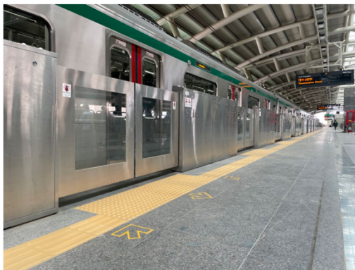
Source: JICA Expert Team Platform Screen Door (PSD)
