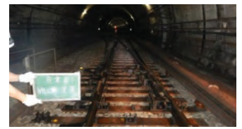
No painted set-off rails with switched position
