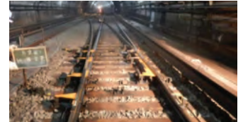
Painted set-off rails with switched position
