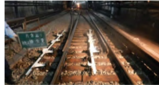
Painted set-off rails with normal position
