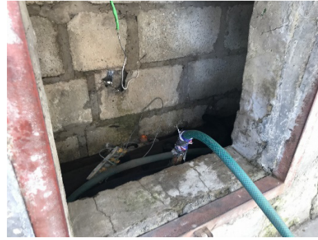
Damaged Water Pipe
