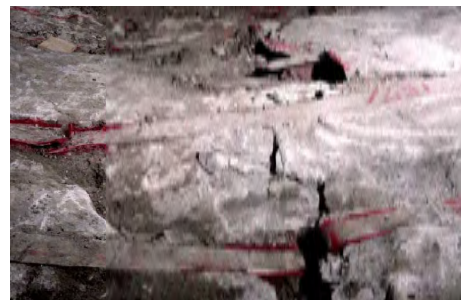
Photo-7 Rupture of Invert Strut
