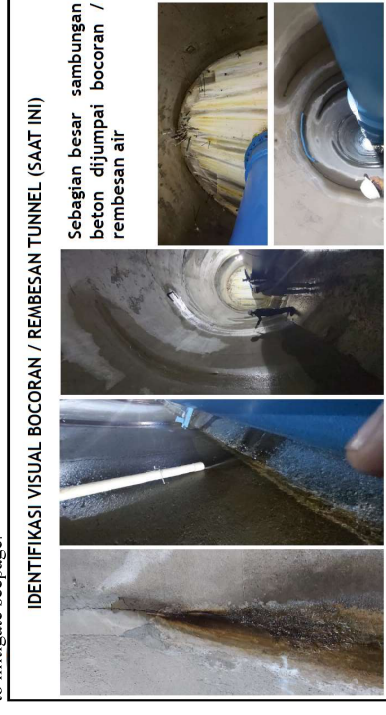
Figure 2: Water leakage at tunnel.
