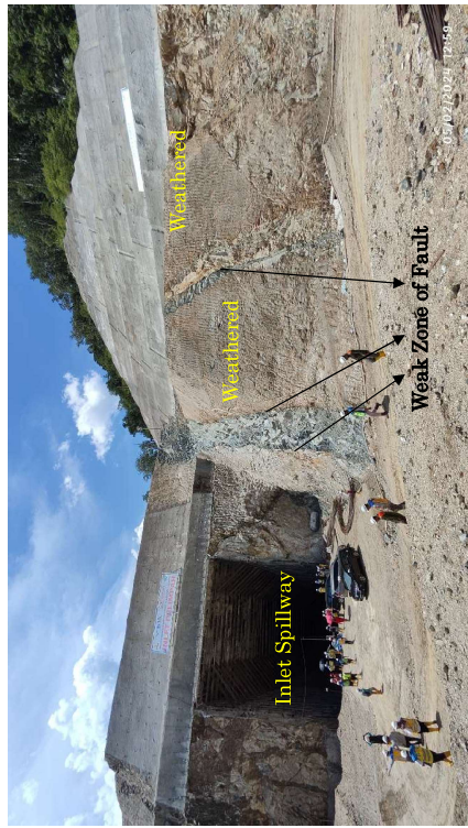
Weathered and fault at the inlet of spillway tunnel
