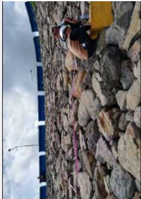
Photo-1 Rip-rap at downstream slopes of the Dam, shows that partially weathered
