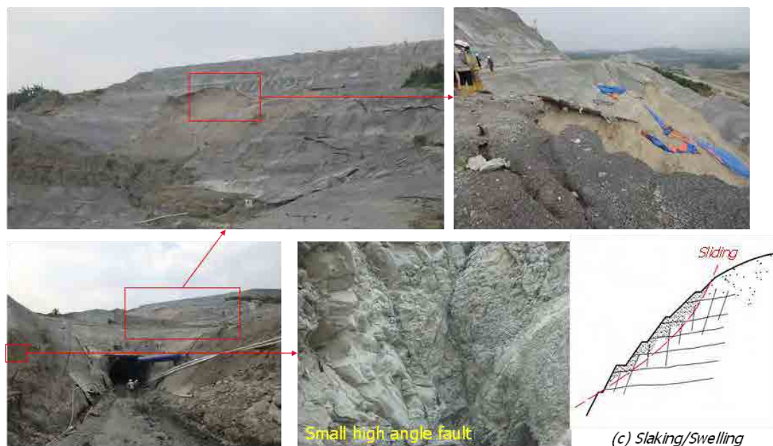
Figure 2.21 Large-scale Sliding Occurred on Cut Slope (Jragung Dam)
