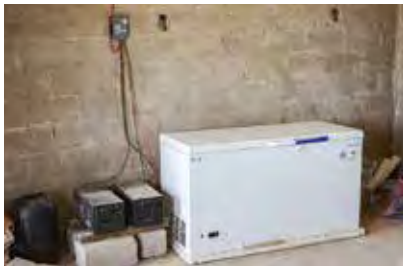
Chest freezer installed in Zula CFC to store fish
