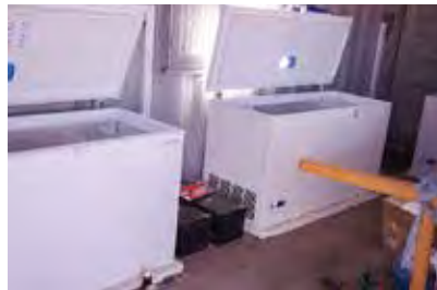
3 Chest freezers Installed in Hirigigo CFC, one is for fish storage and the rest are for ice making
