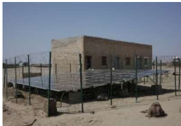
Fig 6-61 Solar panels for ice machine and freezer, surrounded by protective fence facilities
