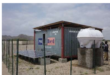
Fig 6-63 Solar system for freezers installed inside the fence.
