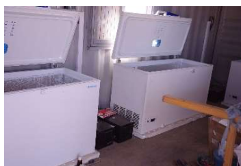
Fig 6-64 Three freezers installed in the Hirgigo CFC
