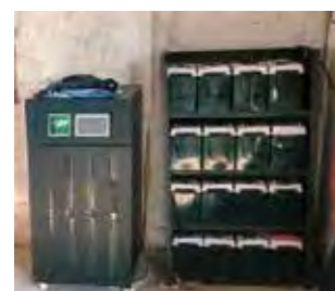
Inverter and 16 pcs of solar batteries
