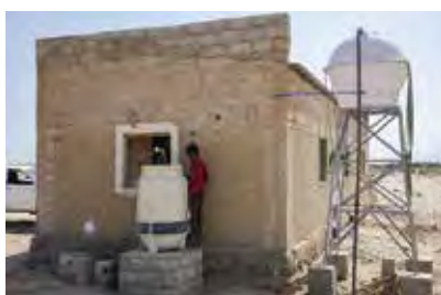
Water cooling tower for condenser cooling, and water tank (2m²) and tower
