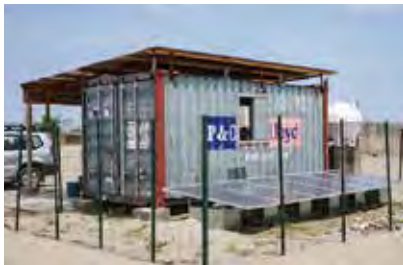
Solar panels installed in Hirigigo CFC
