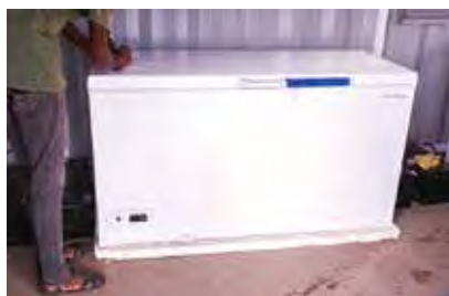
Chest freezers installed in Hirigigo CFC
