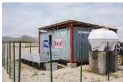
Solar panels and water tank installed in Hirigigo CFC
