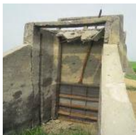
Damaged sluice gate
