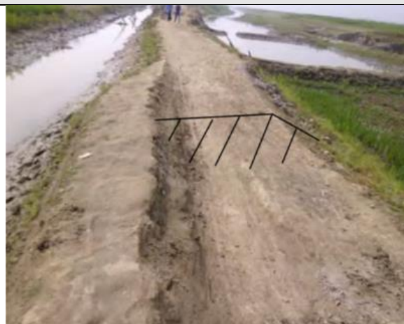
Damage to the submersible embankment due to overflowing water
