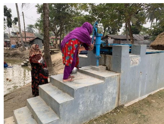
Arsenic iron removal plant
