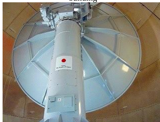
Doppler radar installed inside radar tower in Cox's Bazar
