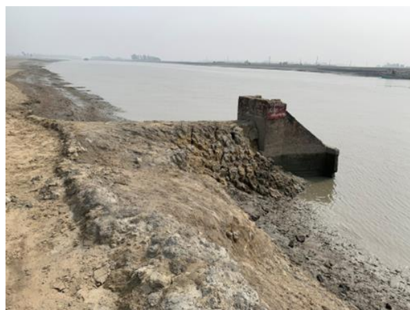
Photo of Matamuhuri River with embankment and abandoned gate
