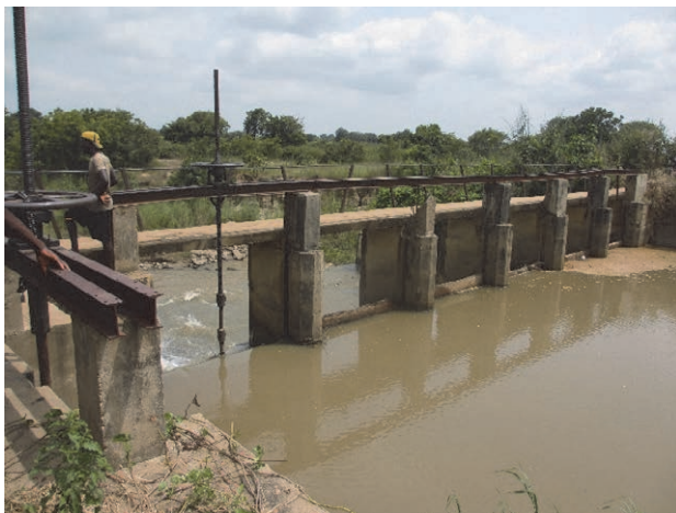
Upstream view, 5 gates lost
