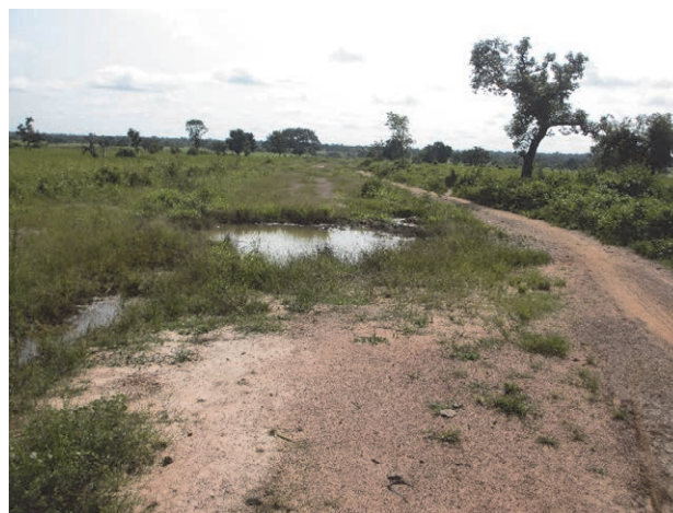
Under construction area. It is difficult for normal vehicles to pass
