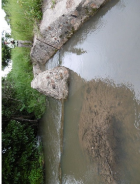
Sedimentation sands at weir shall be removed.
