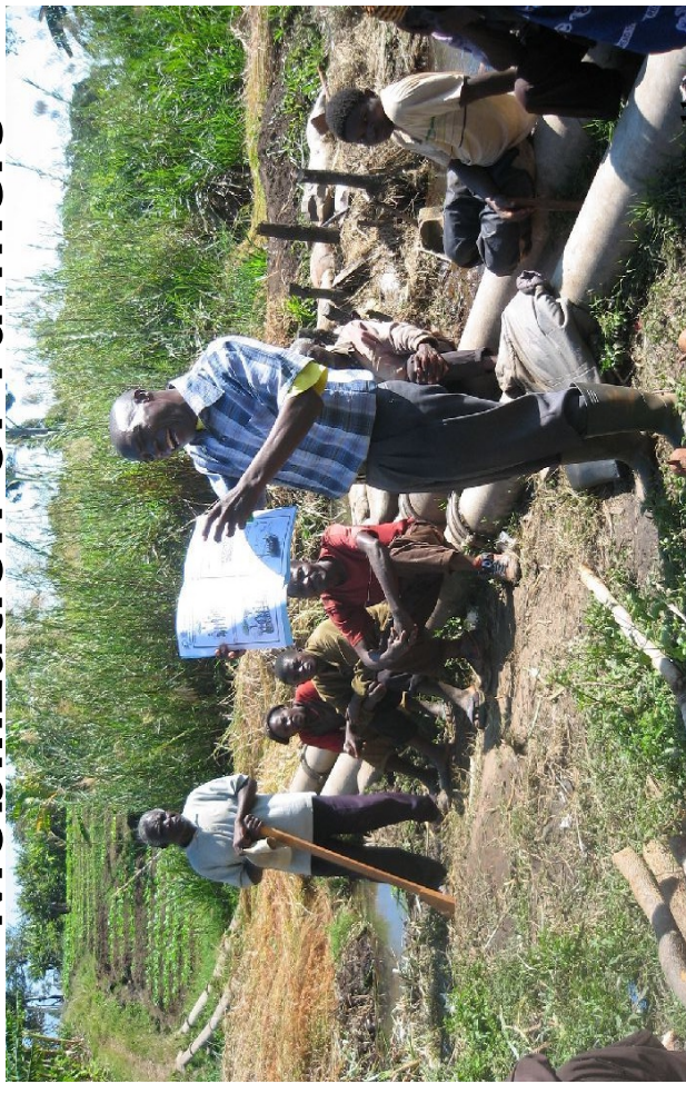
A BEO is teaching the client farmers how to construct the simple weir.
