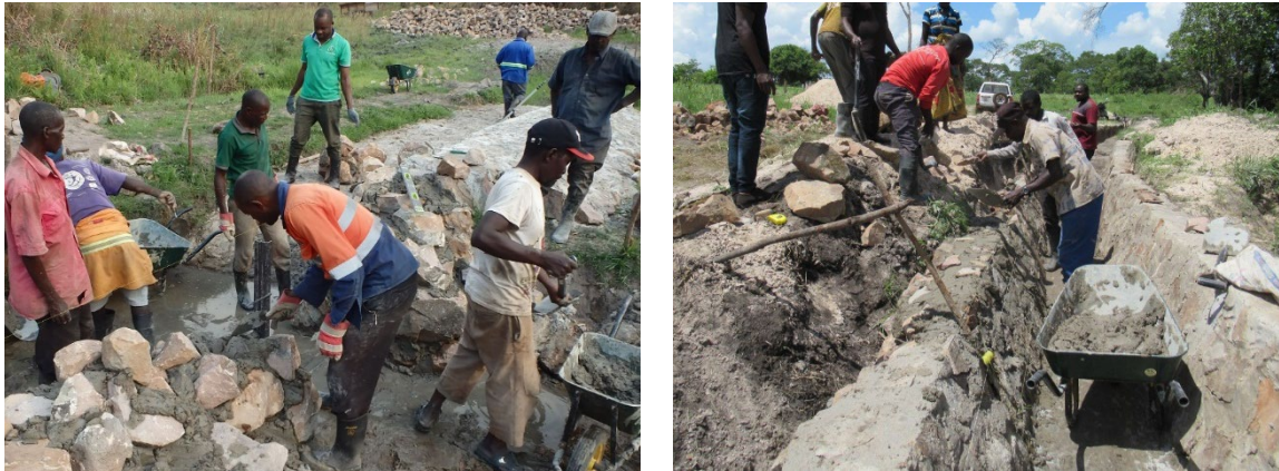
Stone Masonry Works (Left: Weir Body), (Right: Canal) (Kasempa district, North-Western Province)
