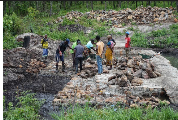
Permanent weir construction (Apr 2022 – Dec 2023) Permanent weir construction was implemented at one site in each of the NT Provinces beginning in 2022. Construction was carried out by farmer group. Japanese experts visited the sites regularly to check progress and provide guidance. (Central Province)
