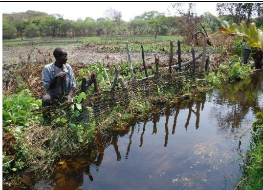
Simple weir (Mwansabombwe) (September 2022) A simple weir at the model site in Mwansabombwe District. At this site, bamboo, which is easily procured locally, was used as the material for the weir. (Luapula Province)
