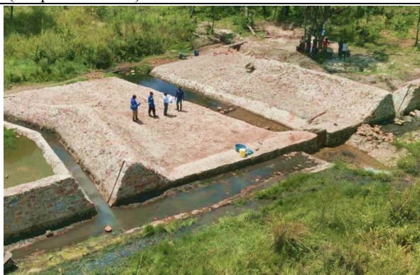
Permanent weir (Kasempa) (December 2023) Permanent weir constructed at the model site in Kasempa. Construction began in the dry season of 2022 and was completed in November 2023. (Northwest Province)
